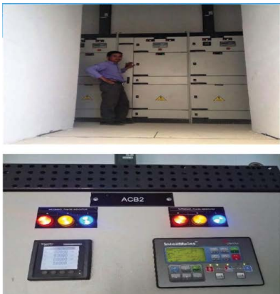
Mobifone Telecommunications Building District 9
