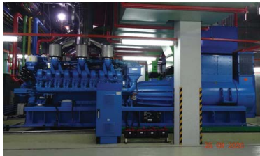
FPT Telecom Data Center
