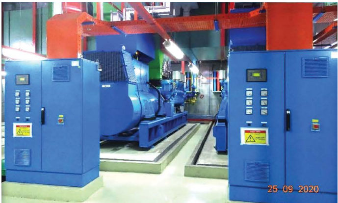
FPT Telecom Data Center
