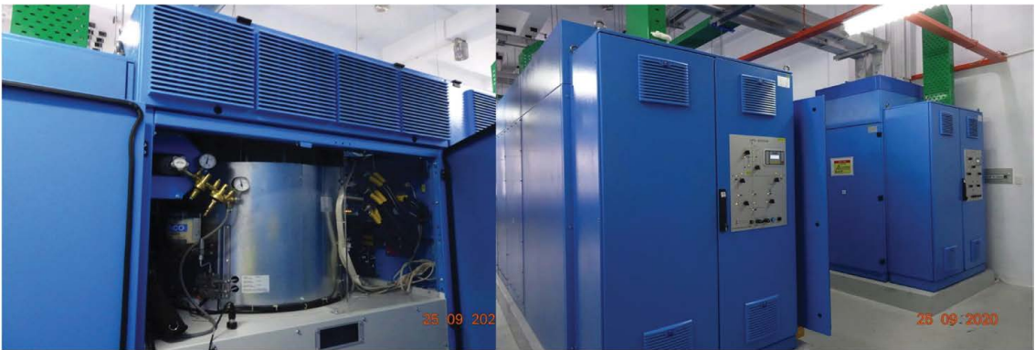
FPT Telecom Data Center
