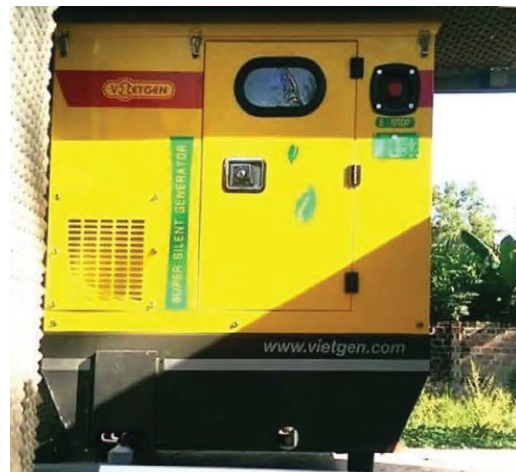
BTS telecommunications station
