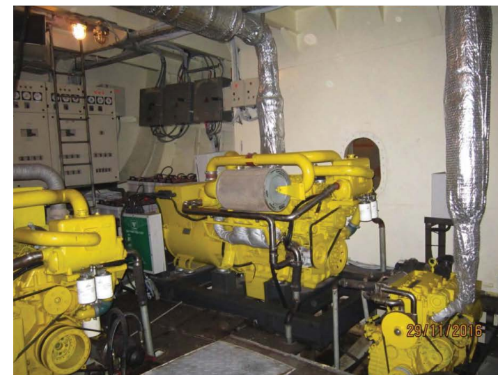
2 generators with 350kVA capacity
