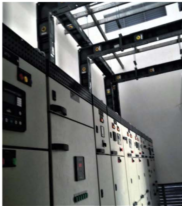
Mobifone Telecommunications Building District 9
