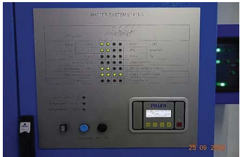
FPT Telecom Data Center
