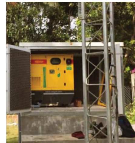
Multiple 8-12kVA generator sets
