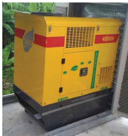
BTS telecommunications station
