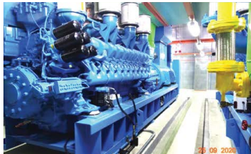
FPT Telecom Data Center
